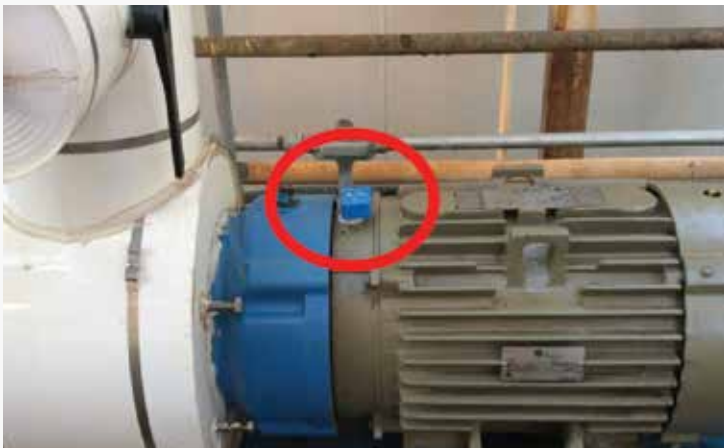
Figure 16: Close coupled motor, mounted over drive end bearing housing
